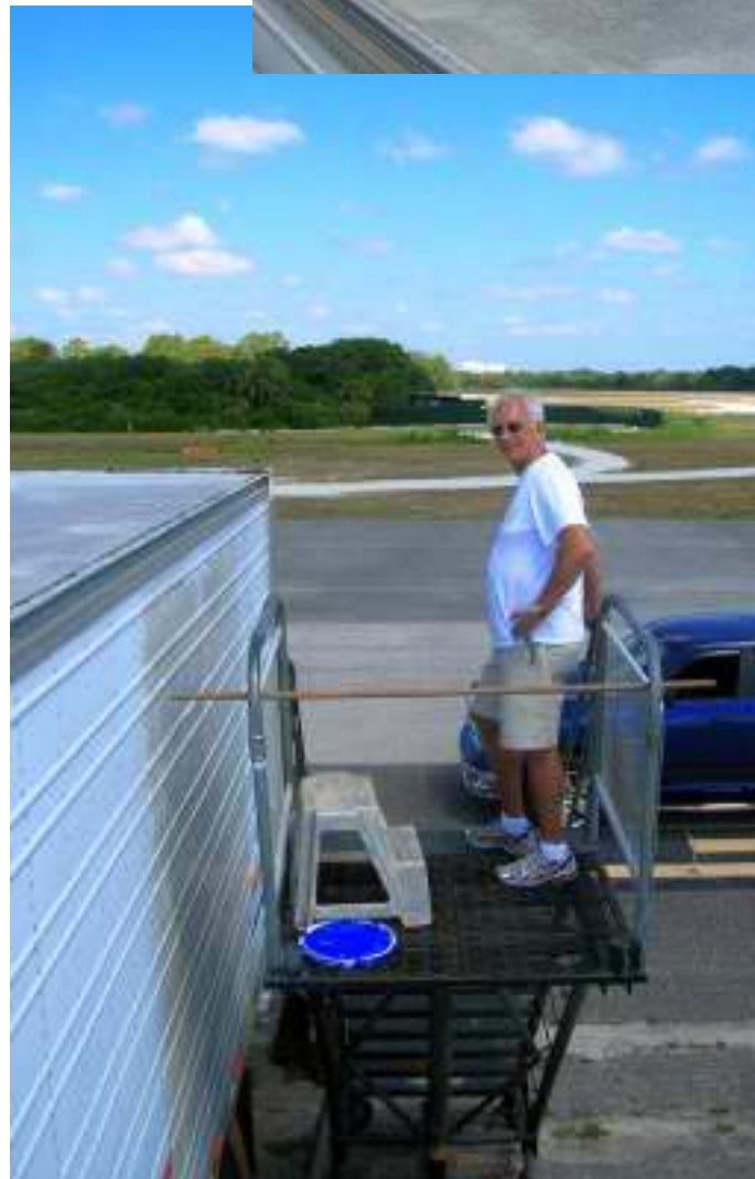
Brad on the semi trailer roof putting down an elastomeric coat to prevent water leaks and to reflect some sun & Ed supervising.
